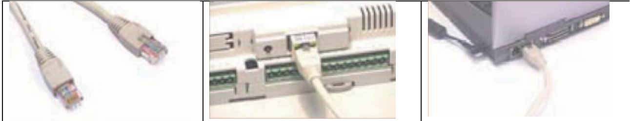
Figure 3.5: demonstration of cable connection to BACNET TCP/IP board
